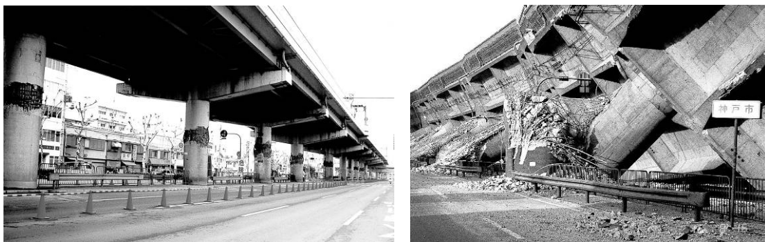
Fig. 1 Flexure-shear Failure of RC Piers in the 1995 Hyogo-ken Nanbu Earthquake The essential reason of the flexure-shear failure was premature termination of the
